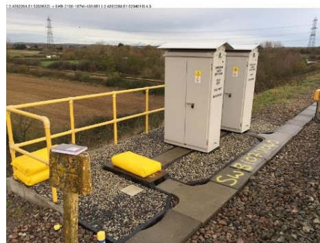
Plate 4.6: An example of LOC Cabinets
