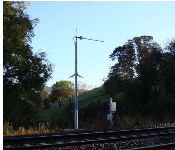
Plate 4.7: A typical pole mounted GSM-R repeater
